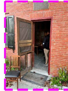
EXISTING CLUB HOUSE REPLACE EXISTING DOOR & ADD HANDICAP PARKING SPACE TO PROVIDE ADA ACCESSIBILITY
